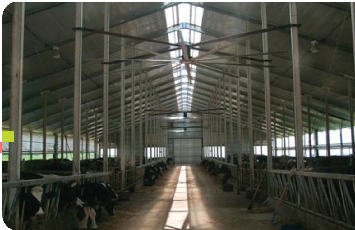
A well-placed HVLS fan is approximately 16 feet off the floor in an area that isn't obstructed by a post, preferably a freestall barn or holding area. Fans should be placed approximately 60 feet apart.
