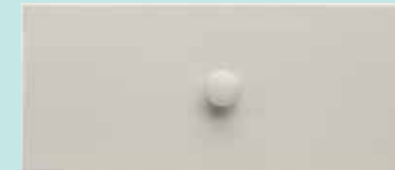
WEATHERED PAINT FINISH
